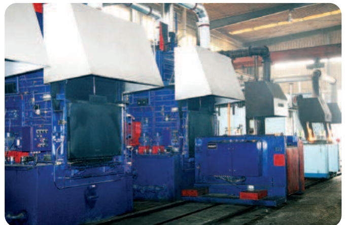
Furnaces for heat treatment process
