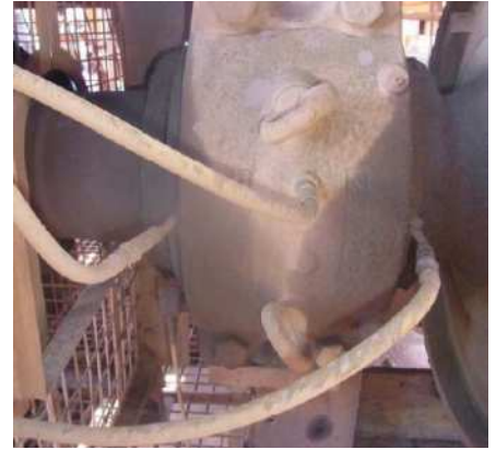
Severely contaminated environment in which the bearing housing assembly operates in.
